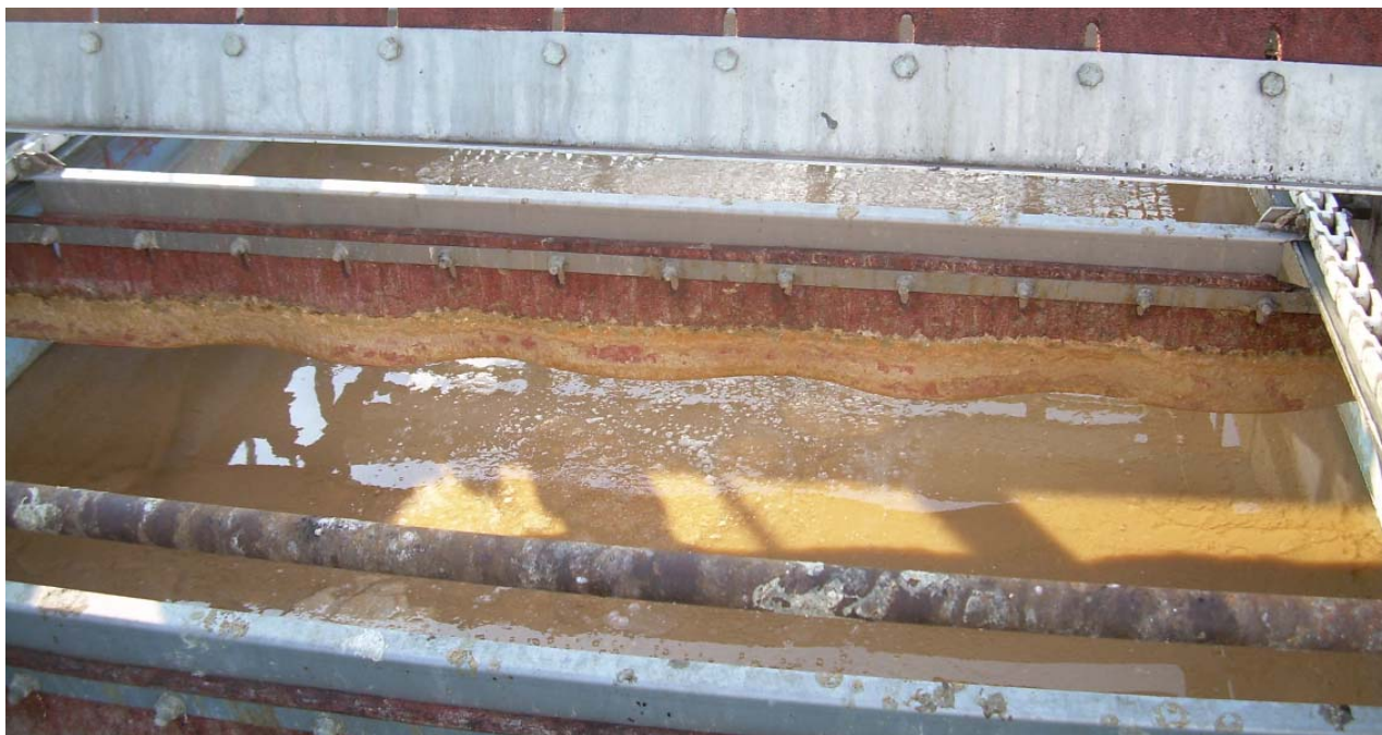
Aspen's wastewater was previously treated through a fat trap that was implemented in 2006. The fat trap has been included as a primary treatment stage for the plant - any fats that are not removed in the fat trap are removed in the DAF Unit
